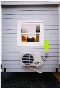
Mini Split Main Shut Off/Disconnect
